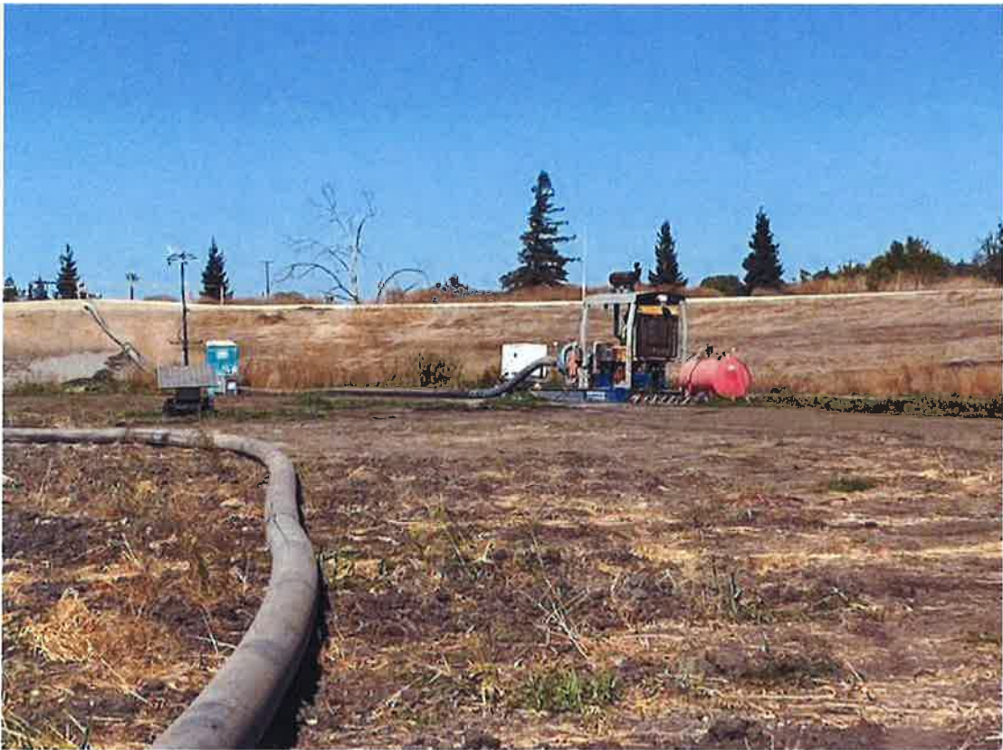
Discharge Pipe Booster Pump on Wright Elmwood Tract
