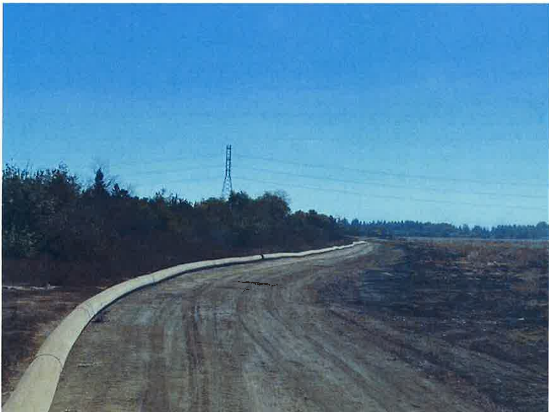
Discharge Pipeline on Wright Elmwood Tract
