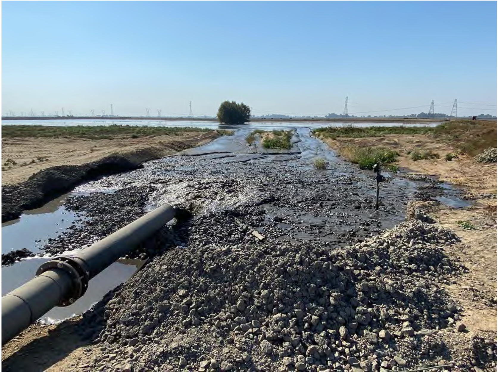
Discharge to Sediment Storage Pond
