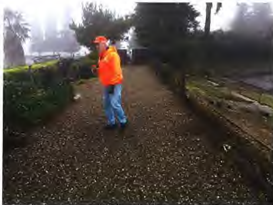
Due to the trimming of the landside hedgerow, the dilapidated eastern third of the old fence has nothing to support it and it has fallen over.
