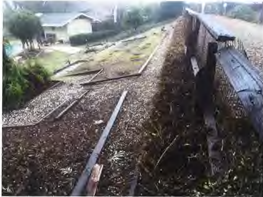
The remaining roots of the old hedgerow along the landside levee crown road hinge point (looking east). Note the dilapidated fence.
