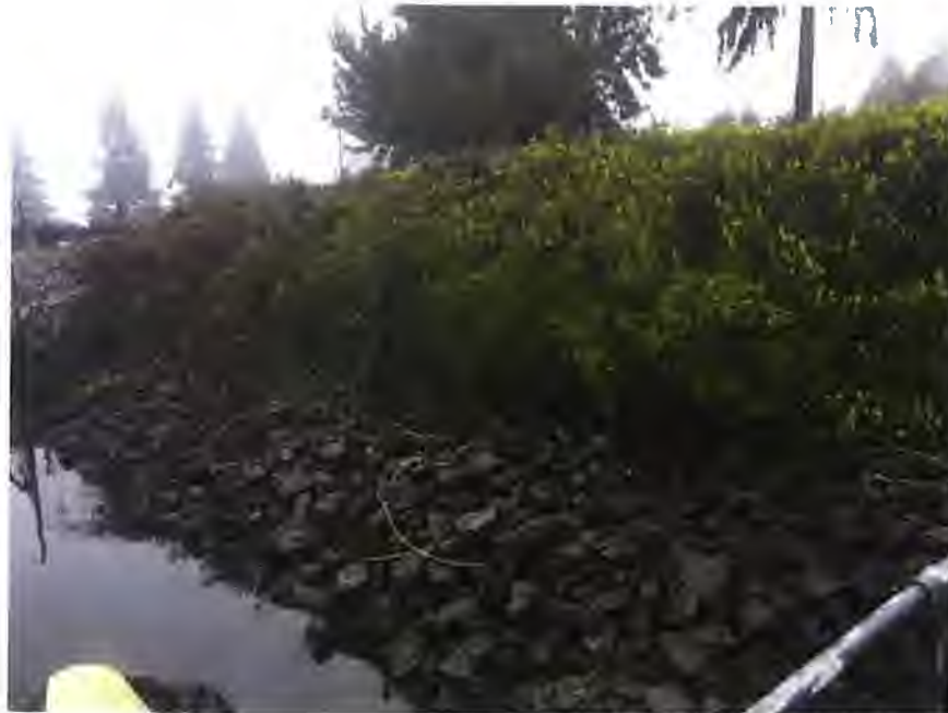
A view of the dense vegetation along the length of the western 75% of the waterside slope, as taken from the boat dock.
