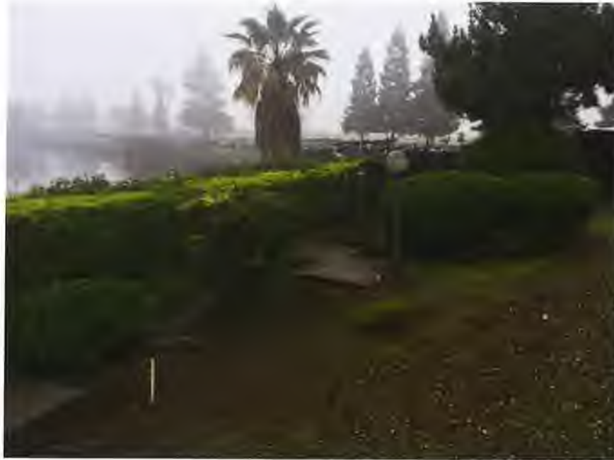
A view westward along the waterside levee crown hinge point at the waterside levee slope. Note the thick hedgerow halfway down the slope that renders the remaining slope un-inspectable.
