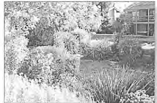
Example of poor vision of levee toe that could hide levee damage.
