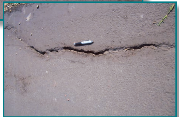
Examples of levee cracks that must be monitored.
