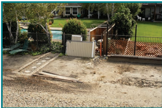
The large piece of plywood and long boards obscure holes or cracks in the levee.
